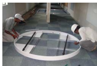
Ceiling on floor!
